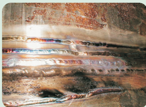
Typical corrosions found on tanks
