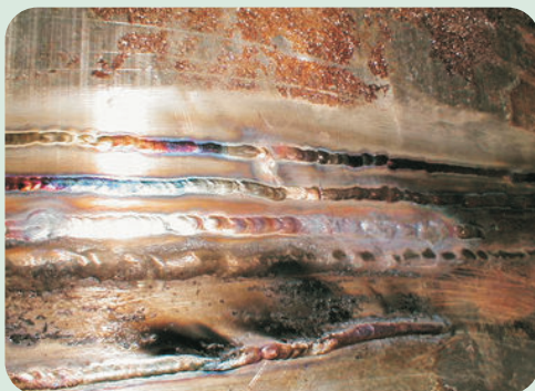
Typical corrosions found on tanks
